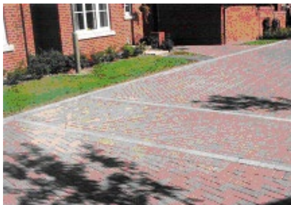
SuDS service crossing
